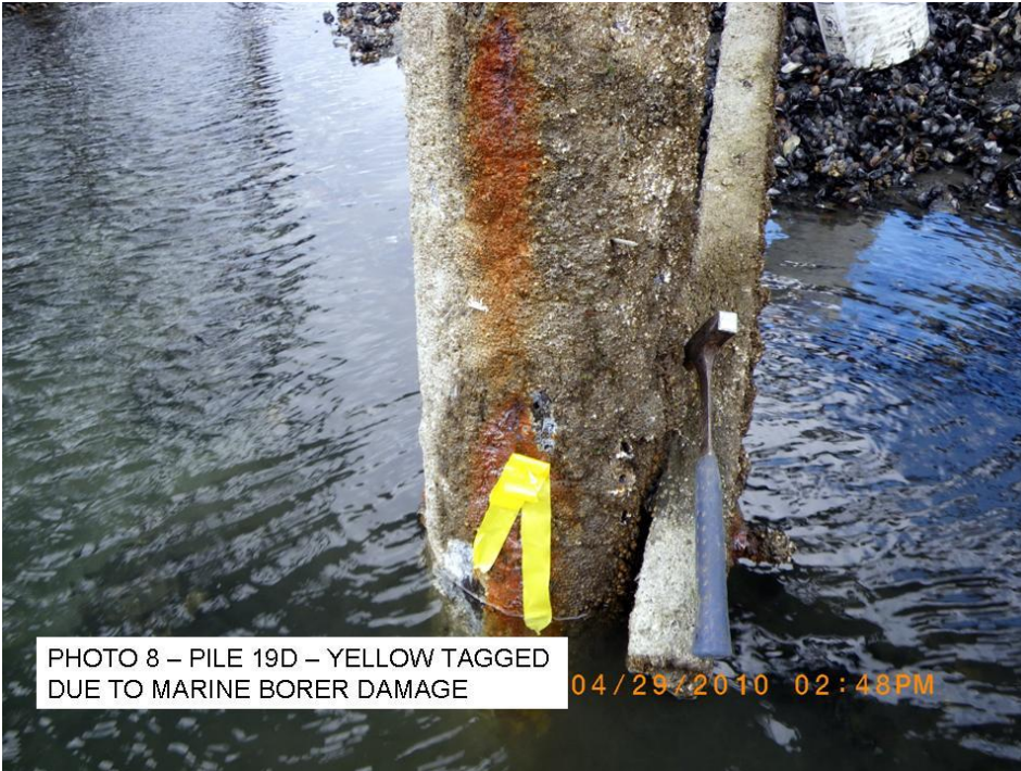
PHOTO 7 – PILE 16D – YELLOW TAGGED DUE TO MARINE BORER DAMAGE
